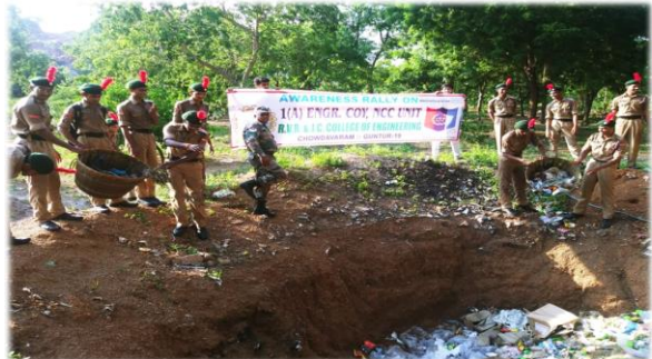
RVR & JC CE, CHOWDAVARAM – 1 (A) ENGR COY NCC, GUNTUR. 24-09-2018 CONSTRUCTING COMPOST PITS - "SWACHHATA HI SEVA"
