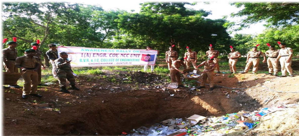
RVR & JC CE, CHOWDAVARAM – 1 (A) ENGR COY NCC, GUNTUR 24-09-2018 CONSTRUCTING COMPOST PITS - “SWACHHATA HI SEVA”
